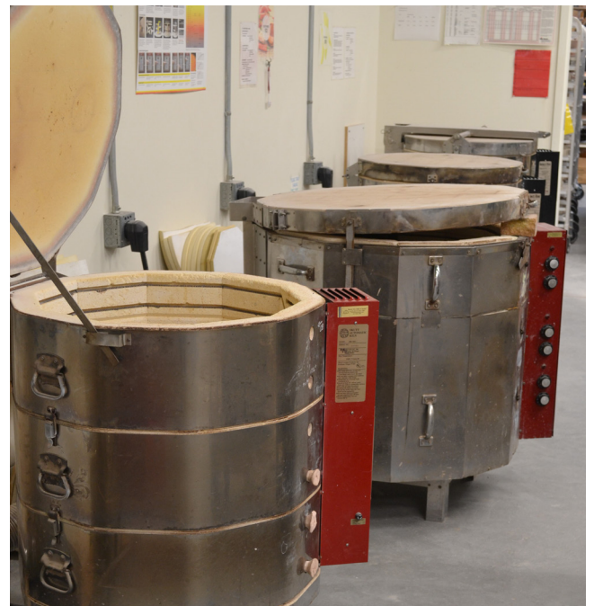
Kiln Room, electric kilns
