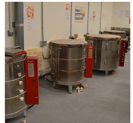
Kiln Room, Electric Kilns
