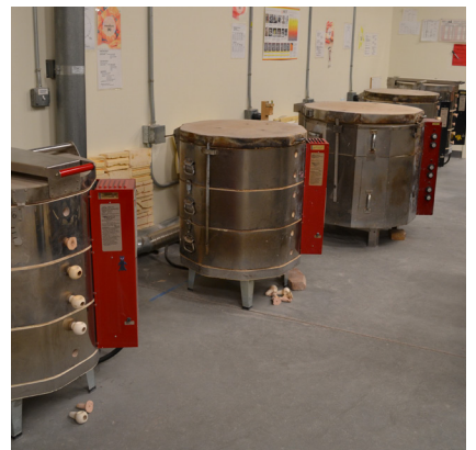
Kiln Room, Electric Kilns
