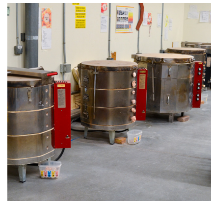
Kiln Room, Electric Kilns
