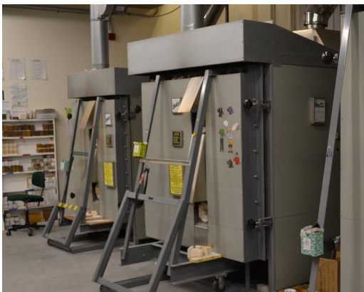
Kiln Room, Gas Kilns
